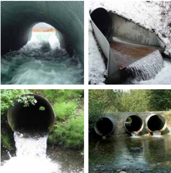
Examples of culverts that do not allow fish passage.
